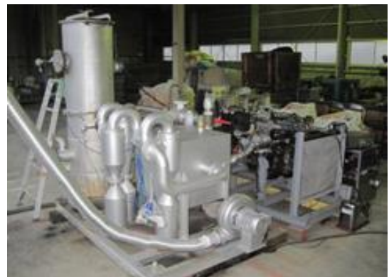
Small woody biomass gasification-power-generation
